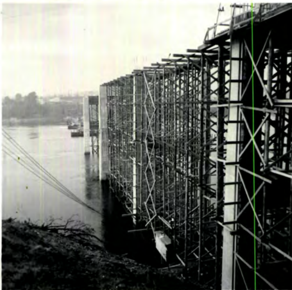
.....DATE: FEBRUARY 26, 1958 REMARKS: Falsework, east side looking South between Piers No. 10 and 8.
